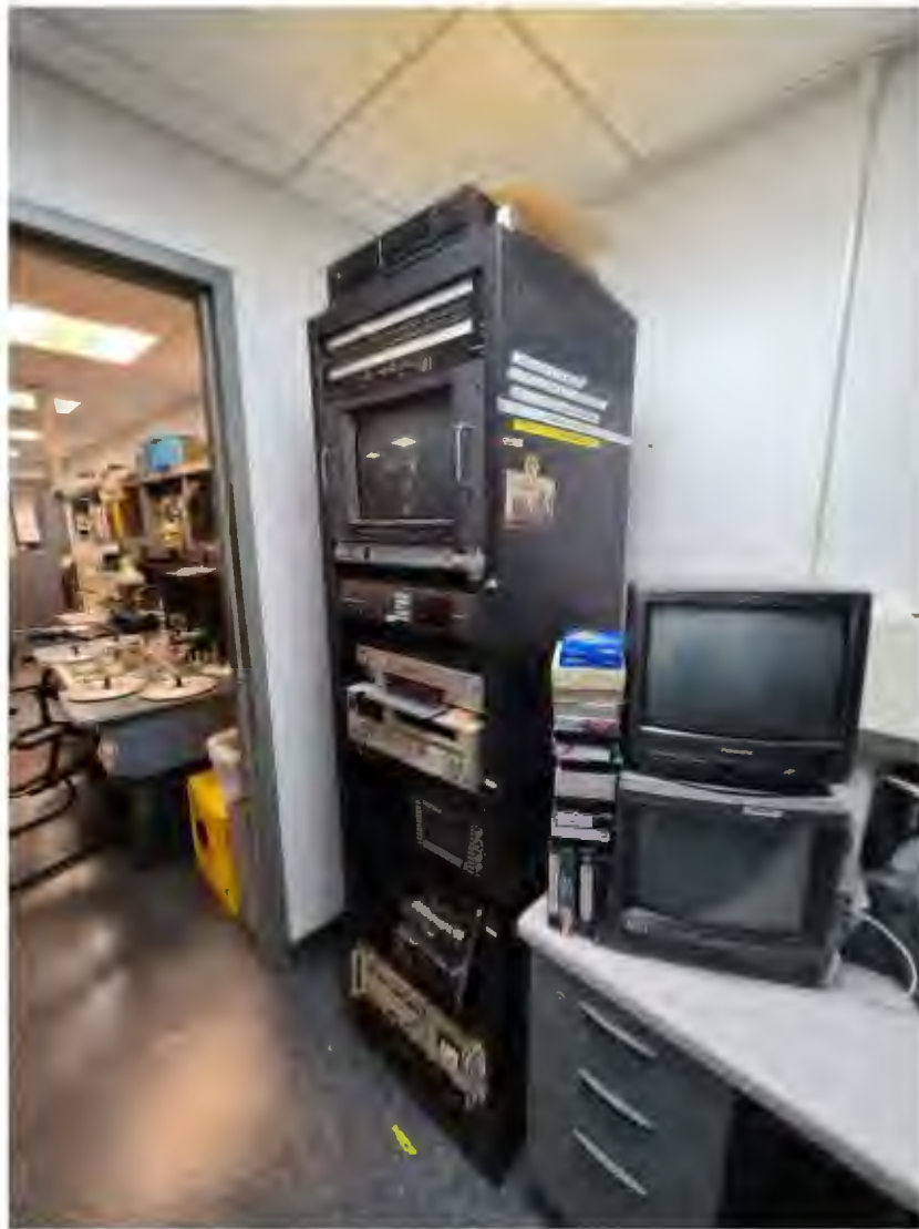
Figure 3: Example of a metal rack. (Dunbar, 2023)
