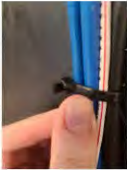
Figure 15: Poorly Cut Zip Tie
